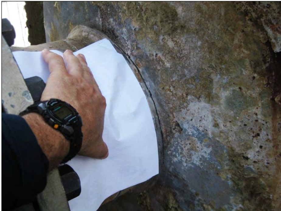
Figure 2: Water hammer damage
